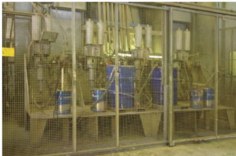
6 – The unit for the electrostatic application of the coatings, inside the insulated cage.
